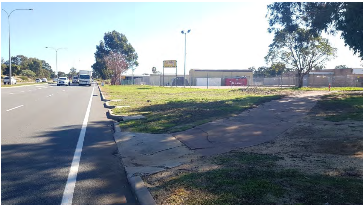
Photo 12: The path connecting Ozich Court to the cycle lanes on Kenwick Link is in poor condition.
