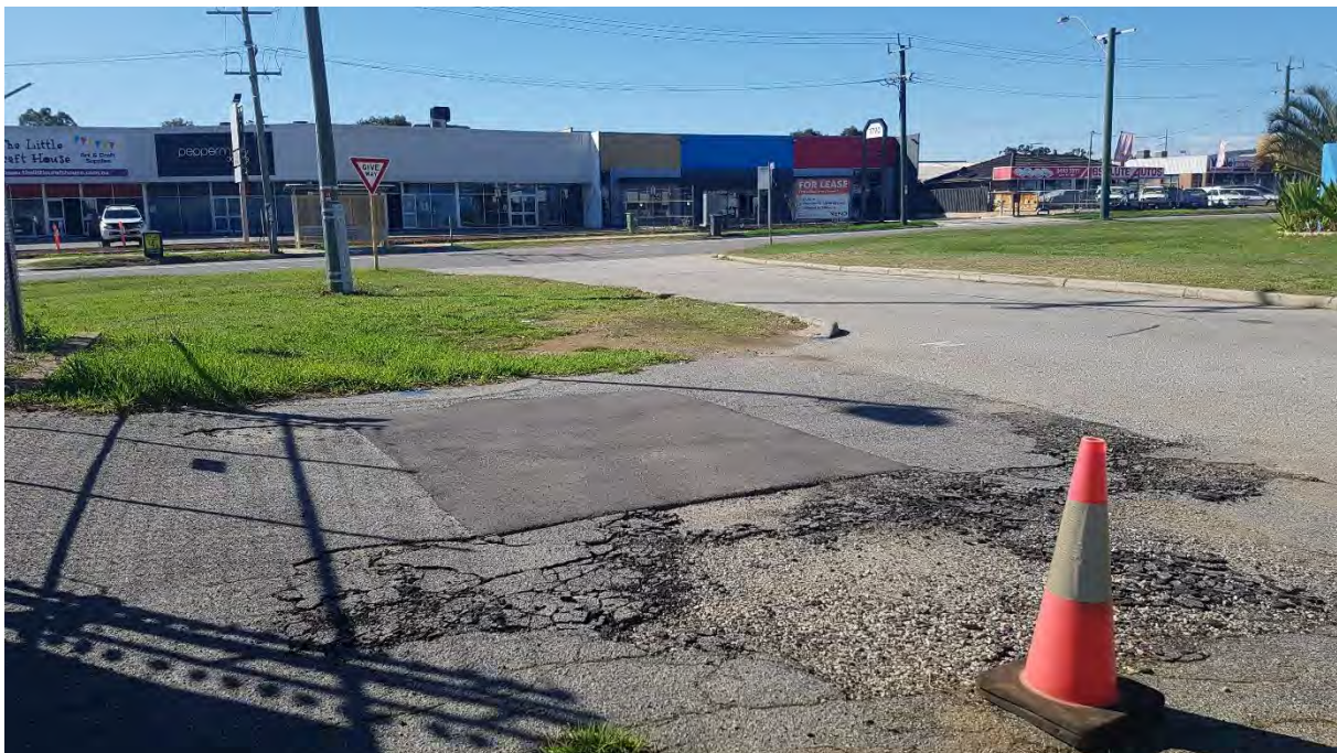
Photo 6: The damaged surfacing of the crossover has been only partly repaired.
